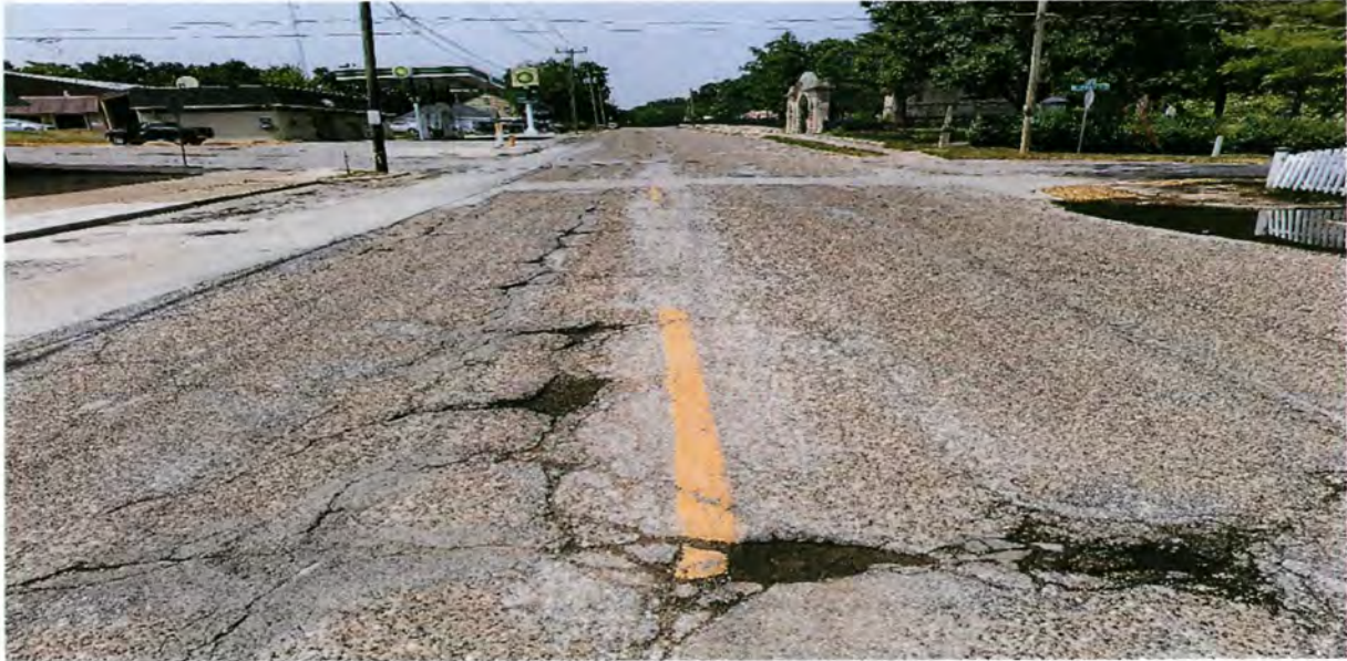
North Court: This form of deterioration can be found throughout the project.
