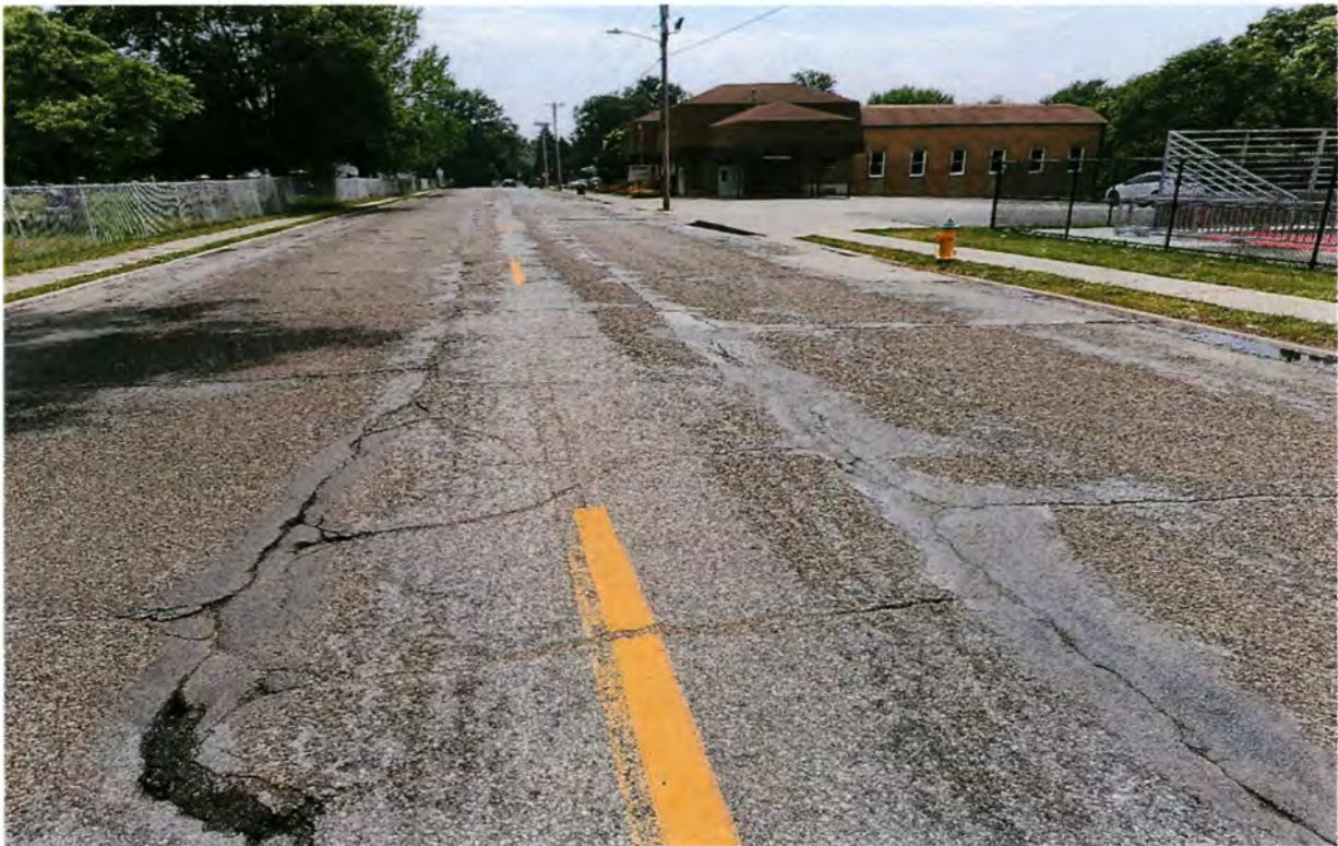
Existing pavement condition. Chip seal was added in the late 90's as an attempt to preserve the asphalt.
