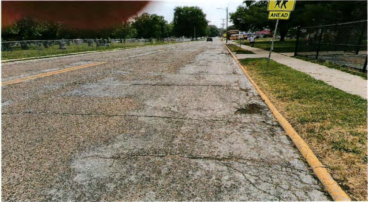
Gutterline failure, existing pavement condition.
