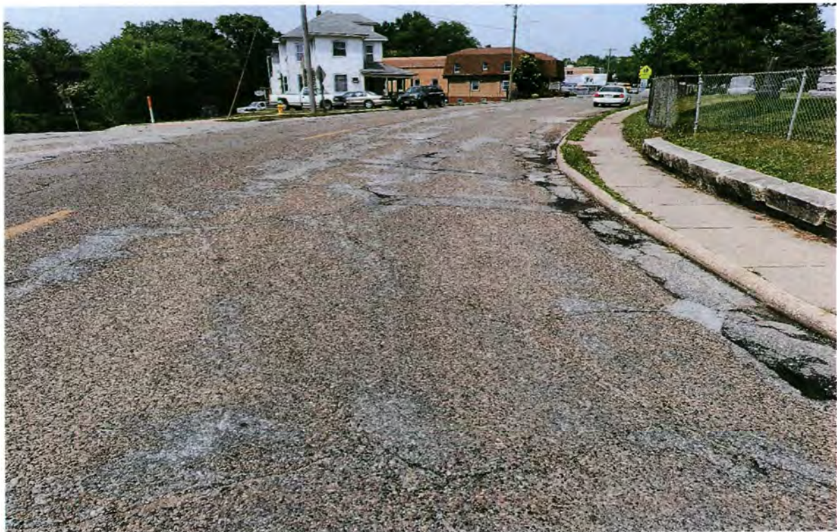
Failing gutterline. Pavement deterioration.
